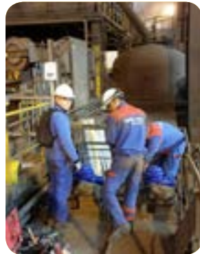
BERNARD CONTROLS team at Arcelor Mittal Steel Dunkerque
